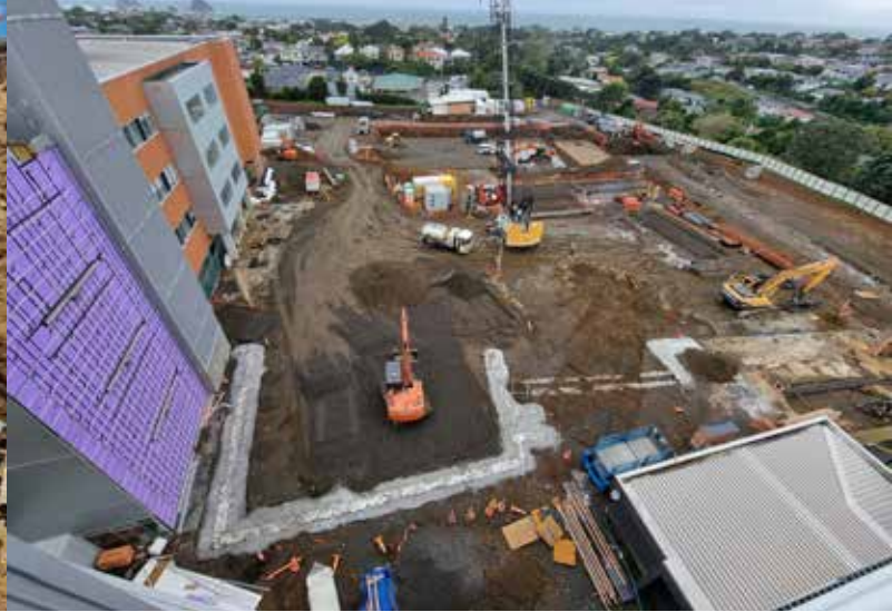
Aerial view of the site with the building outline starting to be visible.
