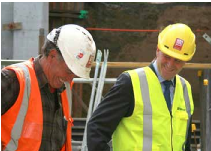
■ Prime Minister John Key (right) during his visit to the Project Maunga Site
