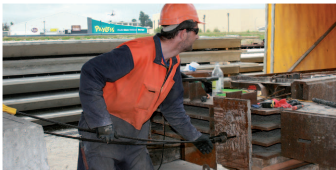
Steel wire is prepared to be tightened before pouring concrete into the Double Tee mould.
