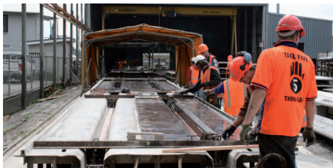
Stahlton workers prepare a Double Tee mould for pouring. On average six of these are produced daily.
