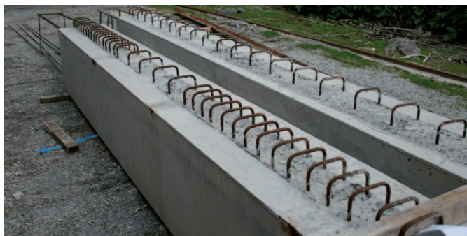
Precast beams which are placed on top of the columns for the flooring units to sit on.
